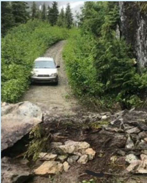
The back end of the Clayton FSR is deactivated. Photo credit: FLNRO
