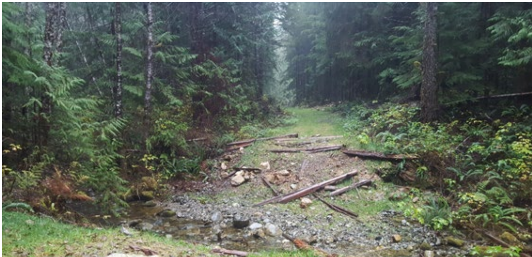
A deactivated FSR and crossing structure in the Alberni Valley. Photo credit: Office of the Auditor General of British Columbia
