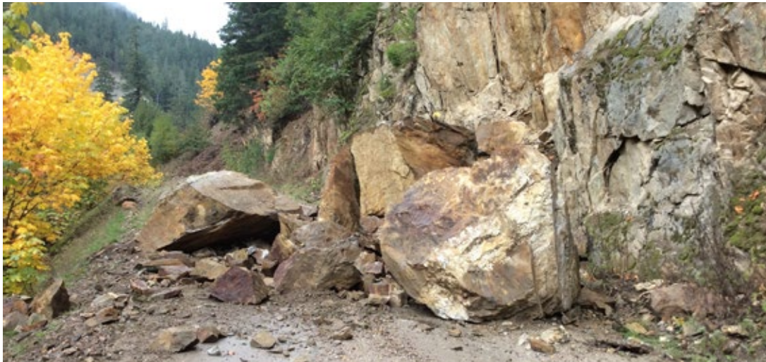
Rock falls can cause safety issues on FSRs. Photo credit: Ministry of Forests, Lands, Natural Resource Operations and Rural Development
