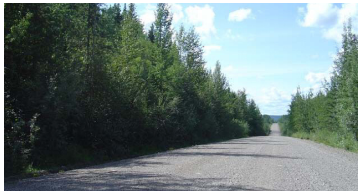
Gravel roads need regular maintenance attention - Auditor General staff photo
