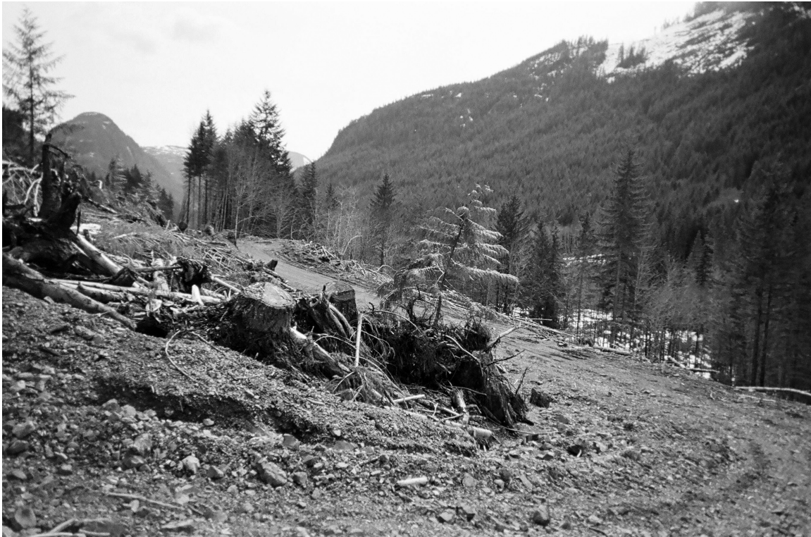
Switchback turn on forest access road. (OAG staff photo)
